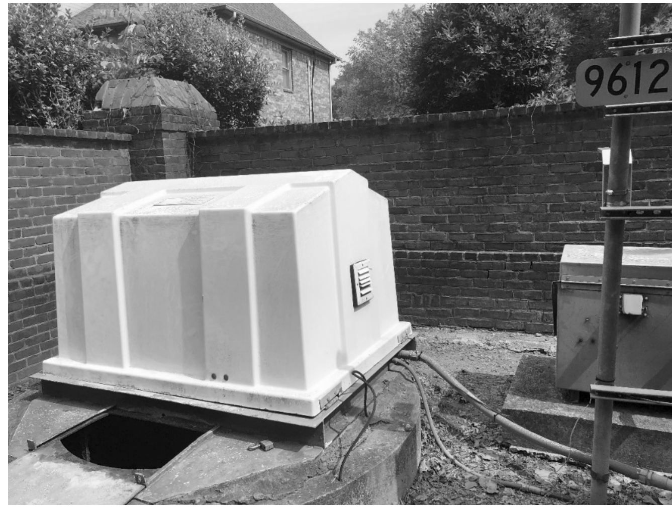
LIFT STATION COVER
