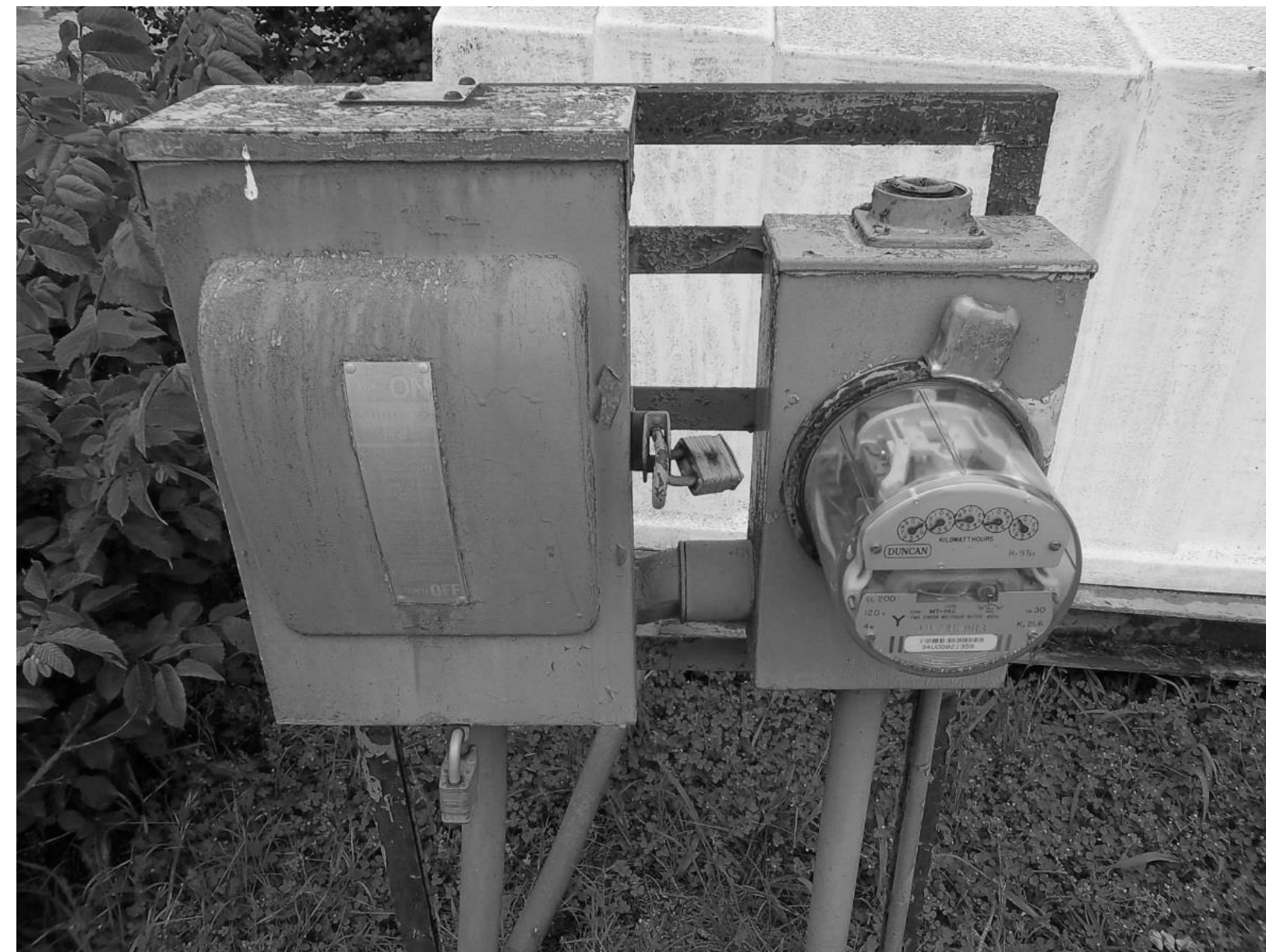
ELECTRICAL SERVICE ENTRANCE
