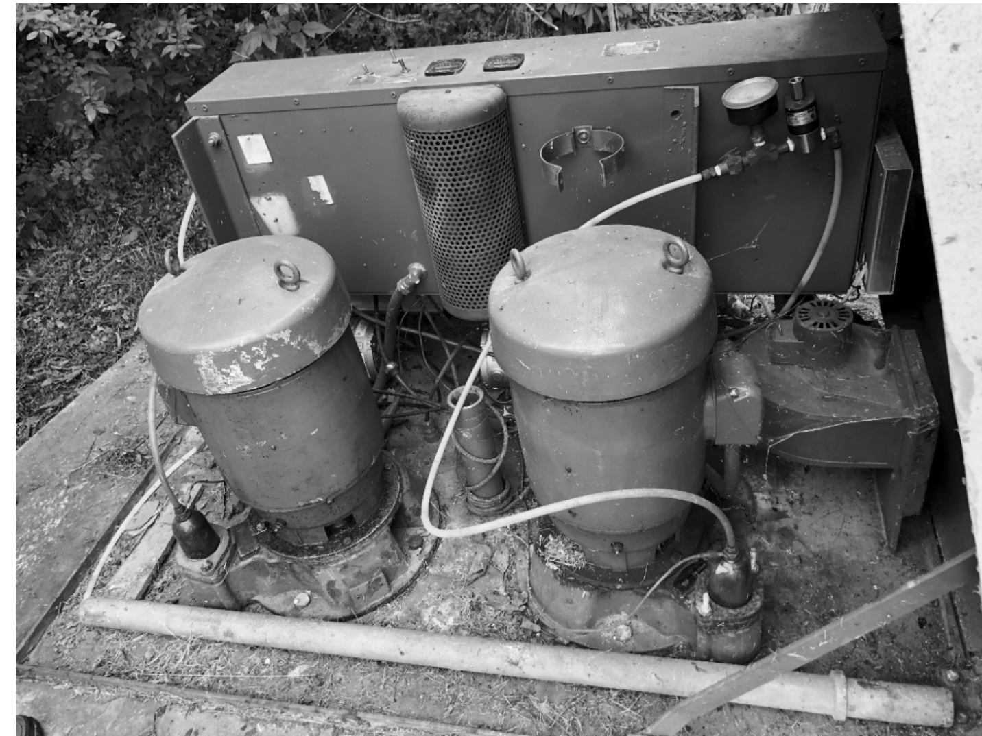
PUMP CONTROLLER MOTORS
