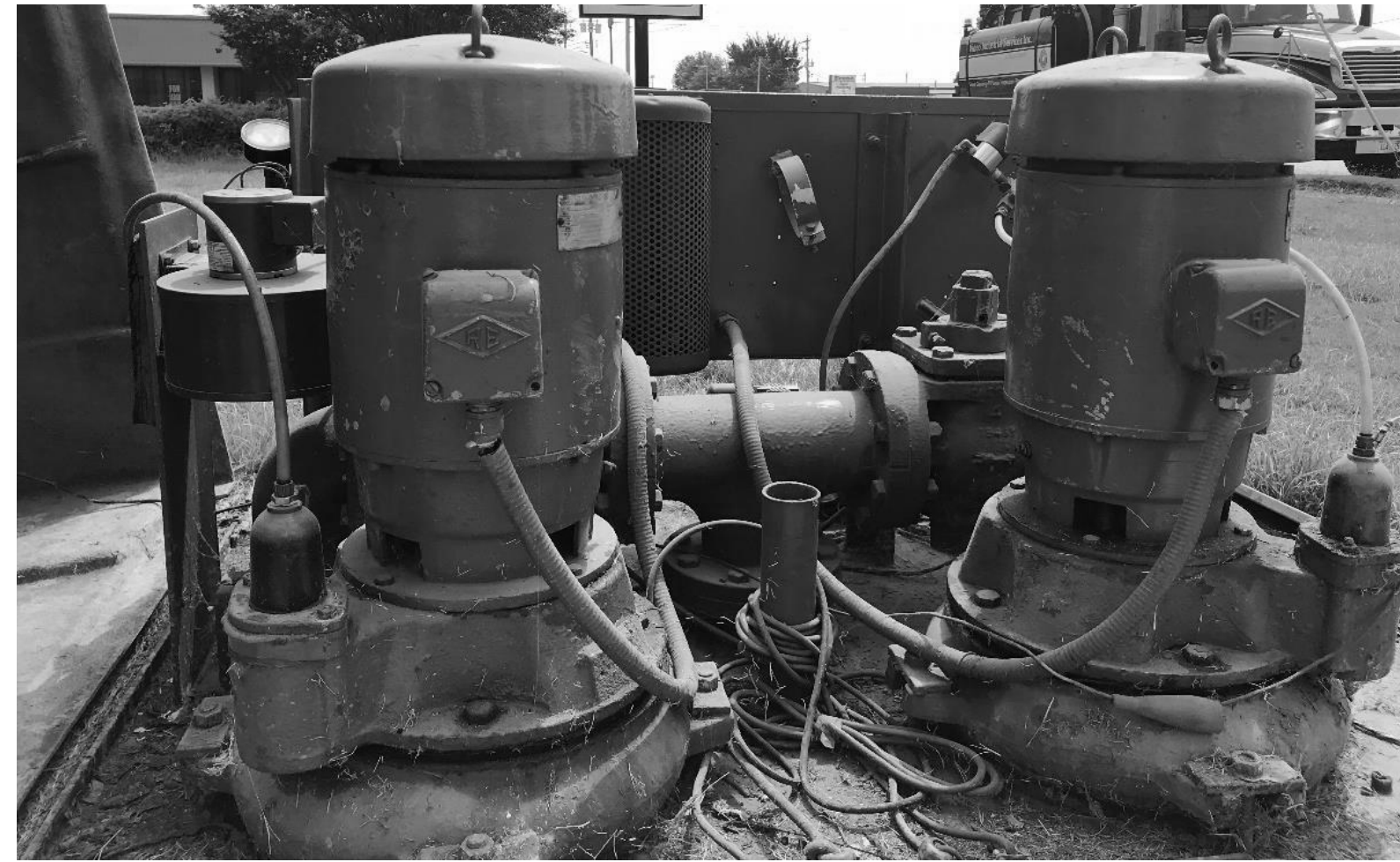
CONTROL PANEL PUMP MOTORS
