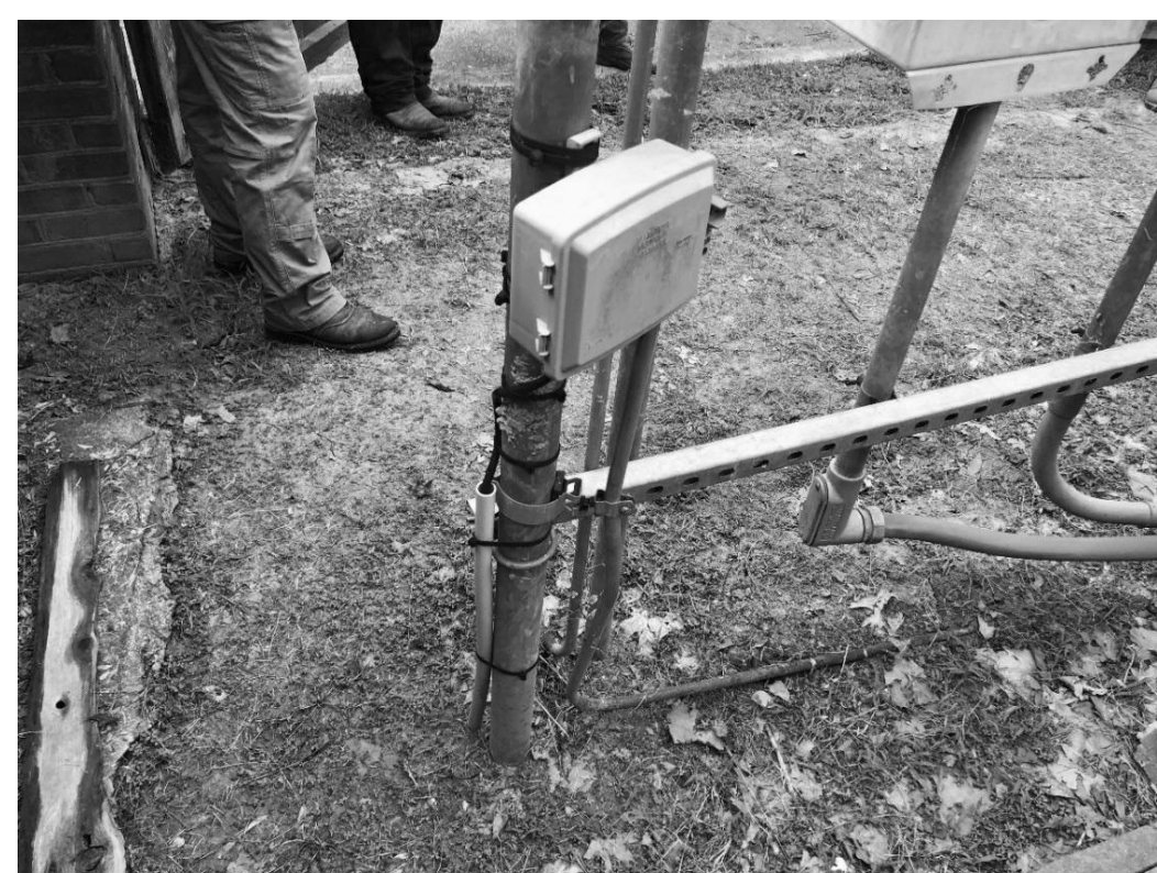
SCADA CONTROL BOX
