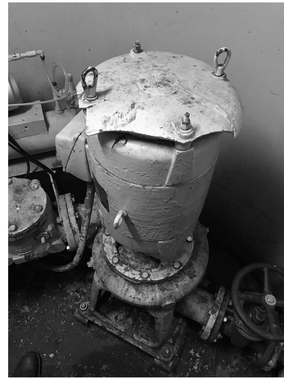
PUMP AND MOTOR
