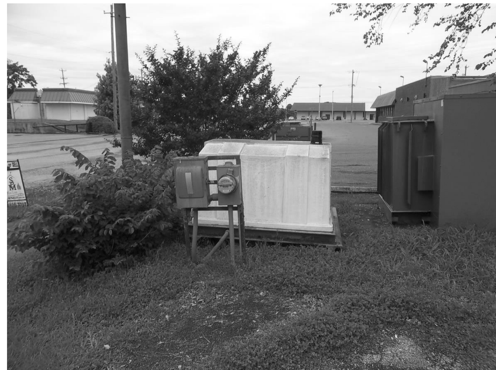
LIFT STATION COVER
