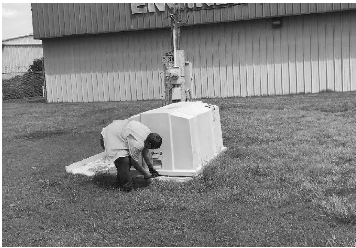
LIFT STATION COVER
