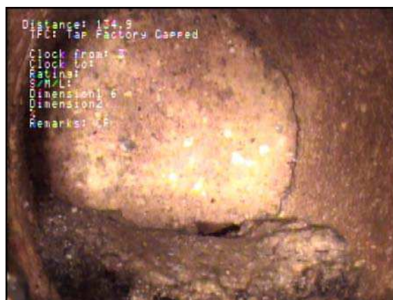
TFC Tap Factory Capped -- CP 134.9 l.f.
