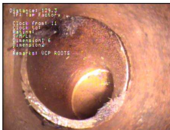
TF Tap Factory -- VCP -- ROOTS 129.3 l.f.
