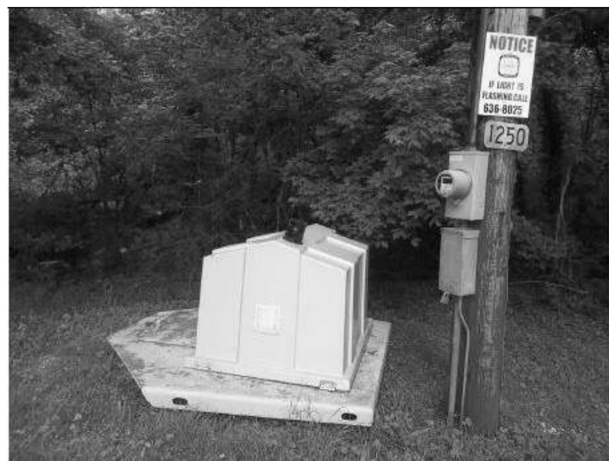
Lift station, warning light, SIGNAGE and electrical equipment.
