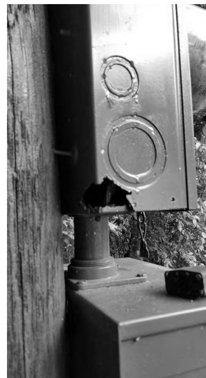
RUSTED HOLE IN METER BASE
