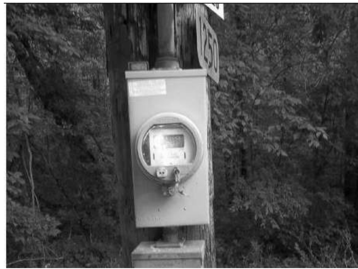
Electrical Meter AND DISCONNECT SWITCH
