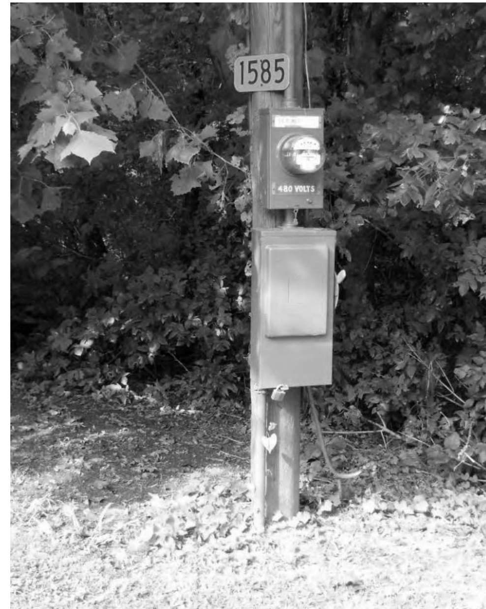
PUMP STATION METER AND DISCONNECT
