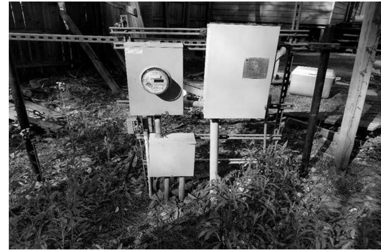
PUMP STATION METER AND DISCONNECT
