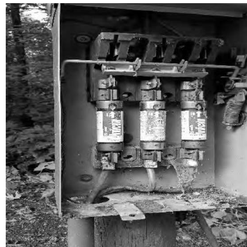
FUSES IN DISCONNECT SWITCH
