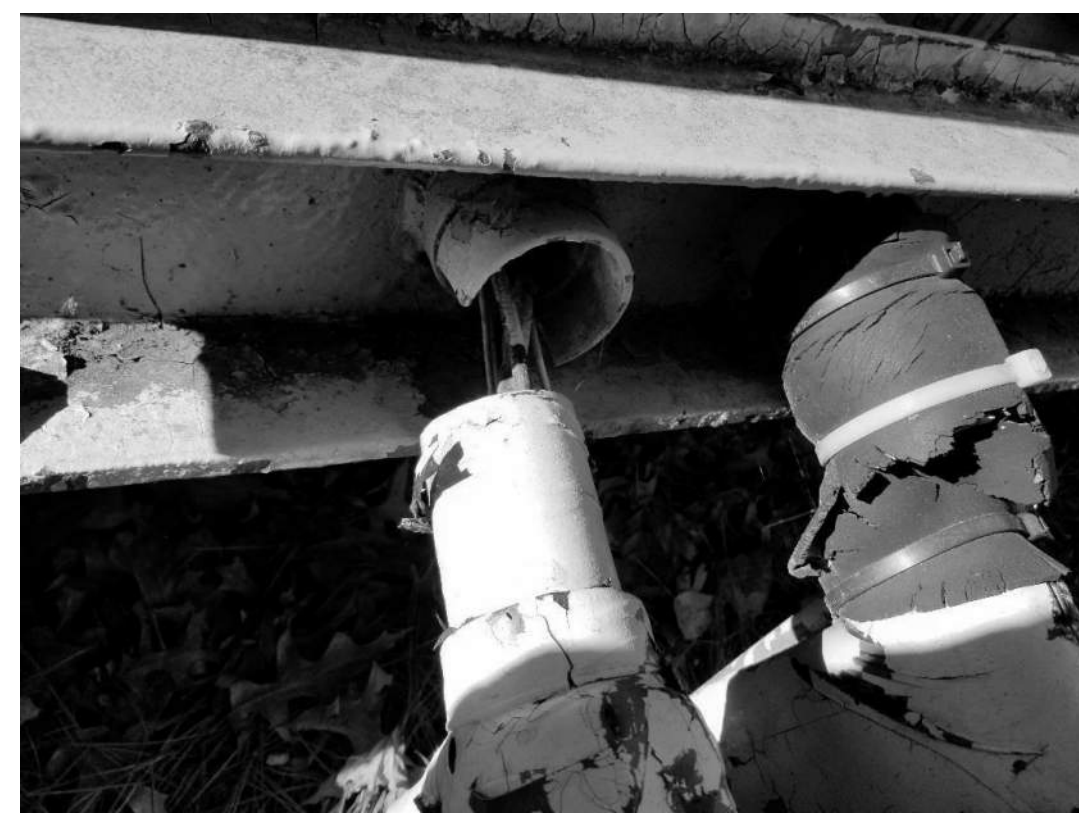
POWER WIRING CONDUIT BROKEN AND IN NEED OF REPAIR
