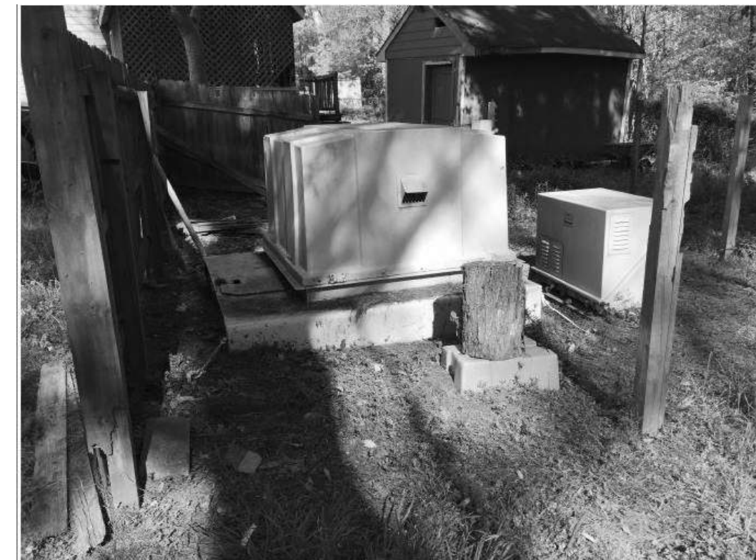
PUMP STATION WITH COVER
