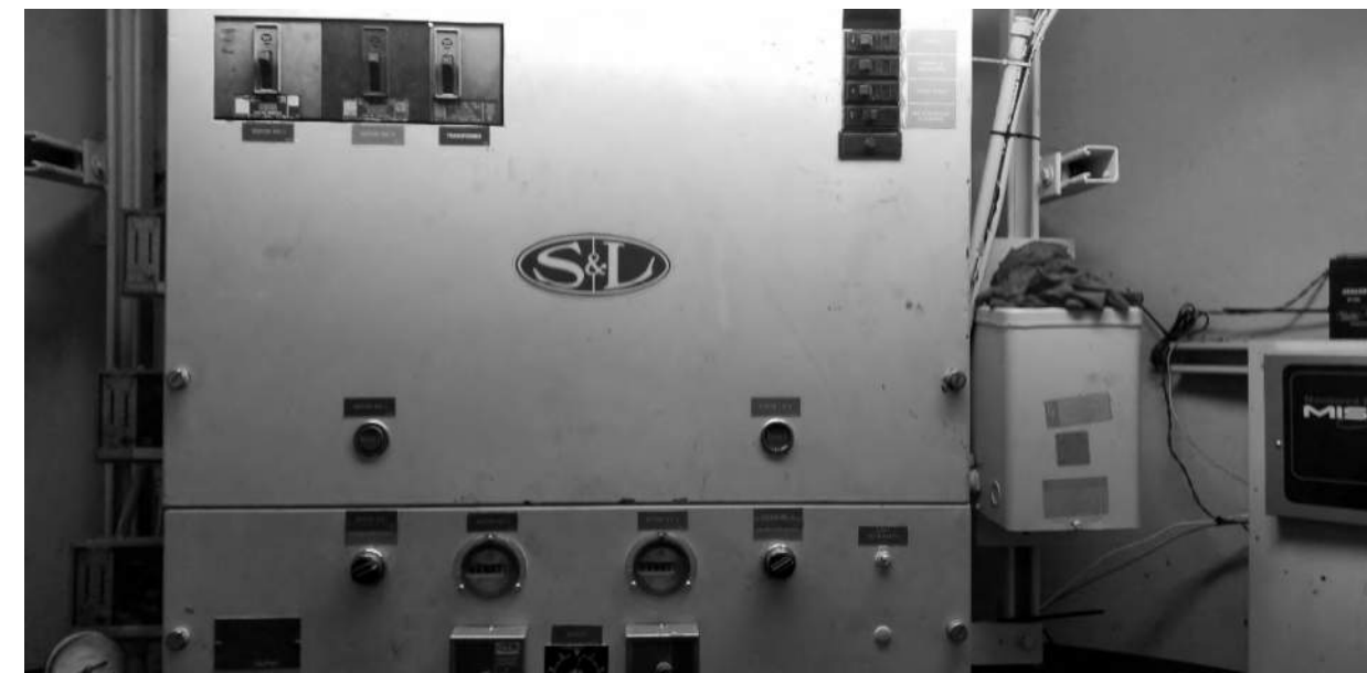
PUMP STATION CONTROL PANEL
