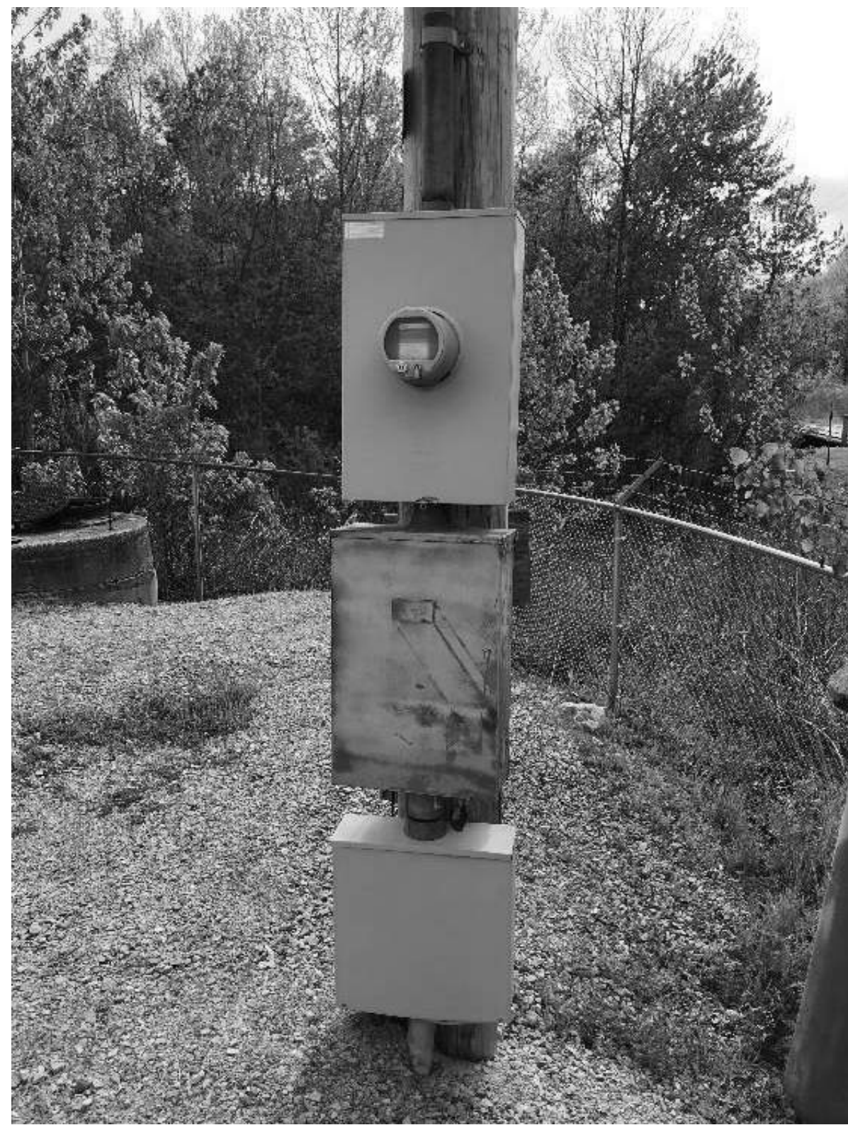
PUMP STATION METER AND DISCONNECT
