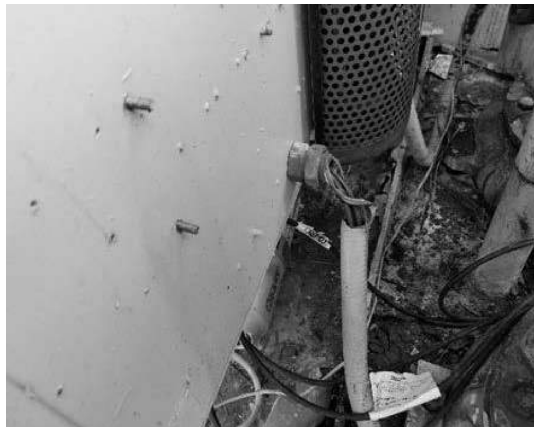
CONTROL WIRING RACEWAY BROKEN AND NEEDS REPAIR
