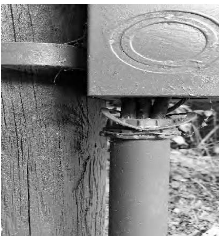
CONDUIT HAS COME LOOSE FROM DISCONNECT
