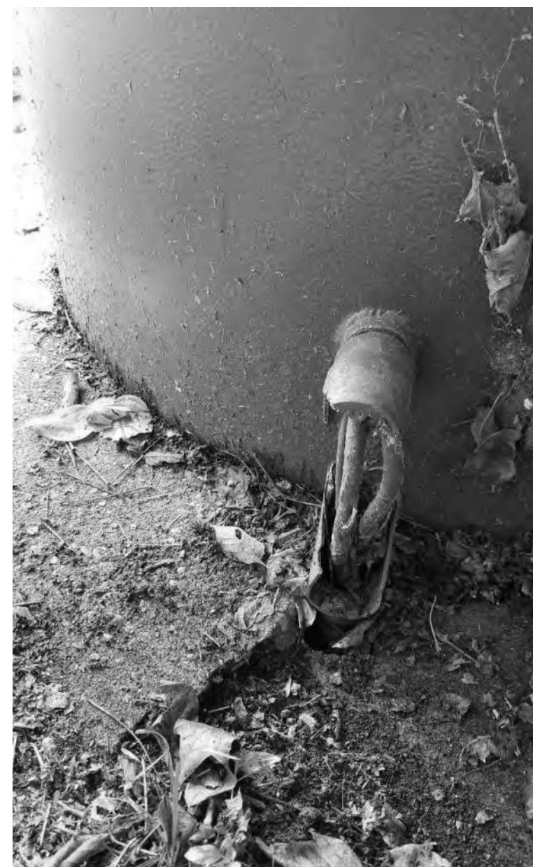
CONDUIT BROKEN AT PIT ENTRANCE
