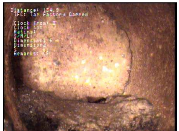
TFC Tap Factory Capped -- CP 134.9 l.f.
