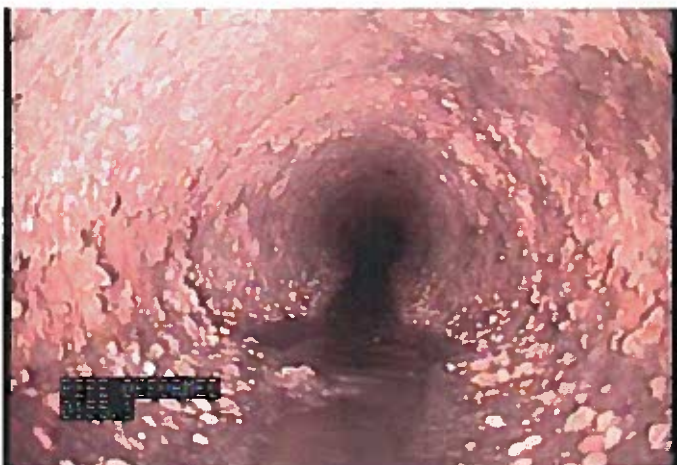
D - Pipe Deformed @ 155.1 ft.
