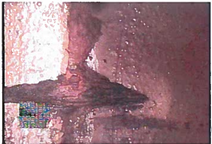
DAZ - Deposits Attached: Other @ 313.3 ft. ENCRUSTATION ATTACHED
