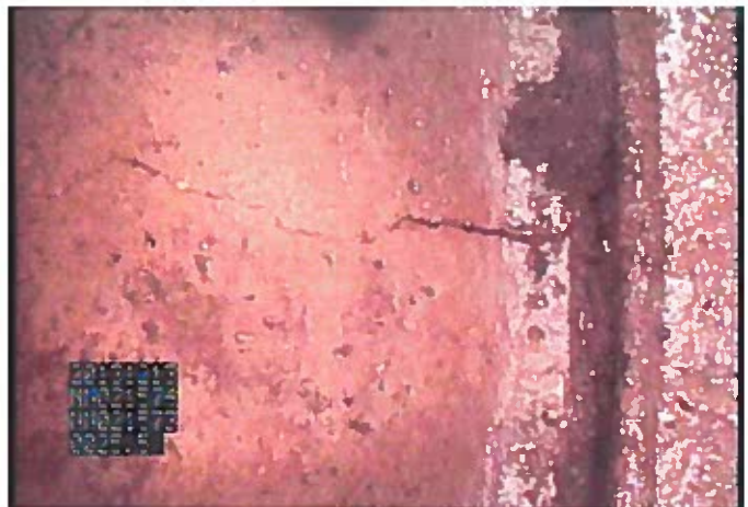
FL - Fracture Longitudinal @ 25.5 ft.
