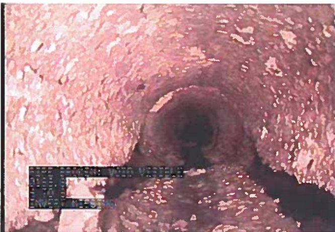
BVV - Pipe Broken: Void Visible @ 188.8 ft. INVERT MISSING
