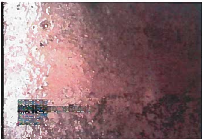
FL - Fracture Longitudinal @ 145.0 ft.
