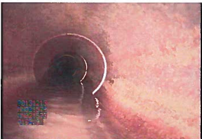
FL - Fracture Longitudinal @ 161.2 ft.
