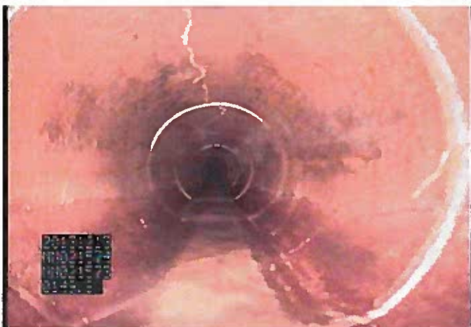
CM - Crack Multiple @ 149.8 ft.
