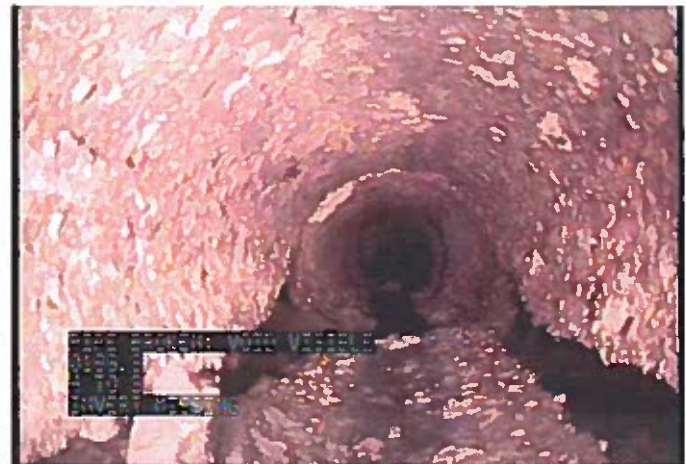
SAP - Surface: Aggregate Projecting @ 188.8 ft.
