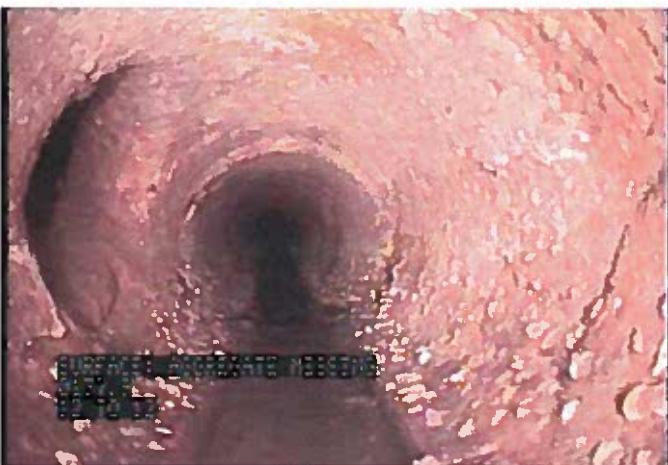
SAM - Surface: Aggregate Missing @ 137.9 ft.
