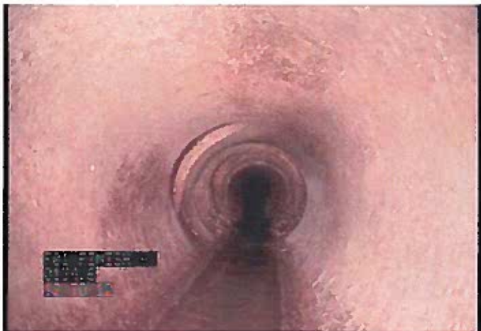
SAM - Surface: Aggregate Missing @ 134.6 ft.
