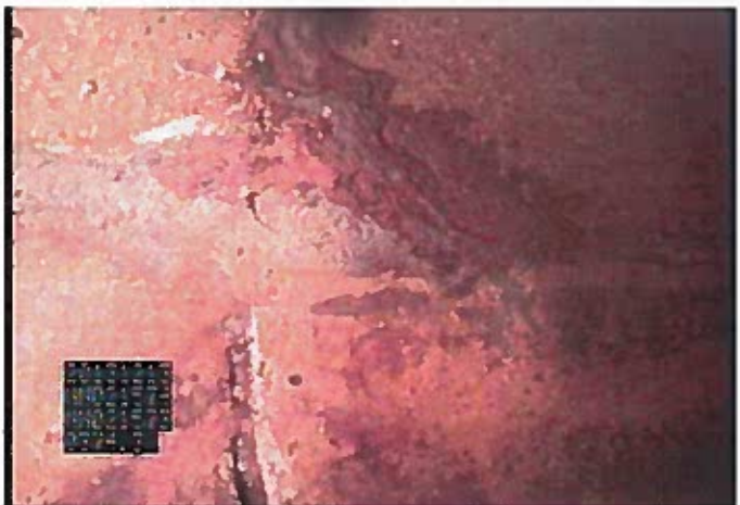
DAE - Deposits Attached: Encrustation @ 374.3 ft.
