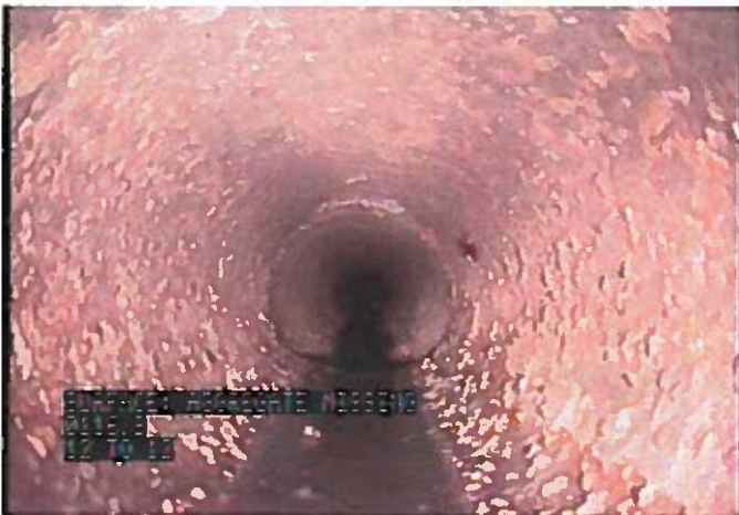
SAM - Surface: Aggregate Missing @ 116.8 ft.
