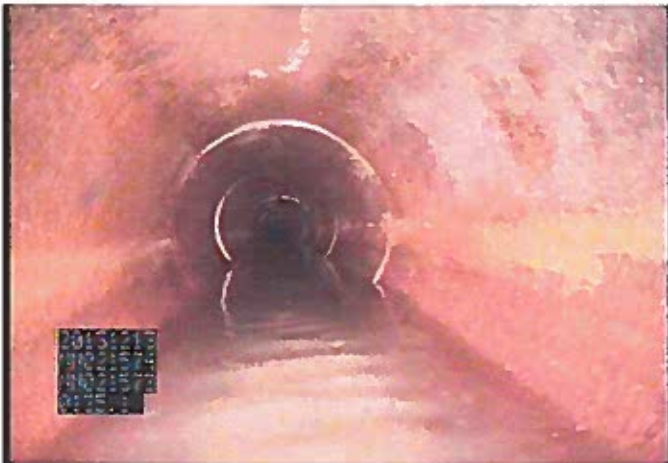
DAGS - Deposits Attached: Grease @ 135.1 ft.
