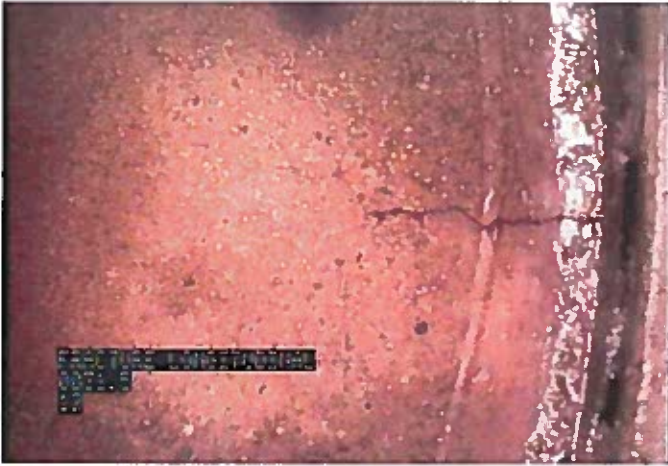
CL - Crack Longitudinal @ 31.5 ft.
