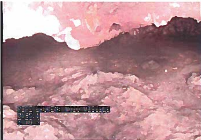
BVV - Pipe Broken: Void Visible @ 185.1 ft.
