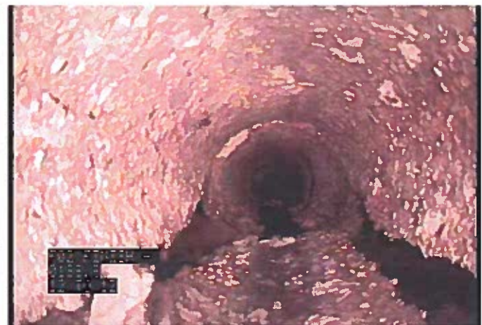
SAM - Surface: Aggregate Missing @ 188.8 ft.
